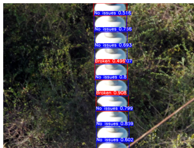
Figure 6. Representative detection outputs on real UAV inspection images. Bounding boxes illustrate predicted defect instances across the four target classes. The examples demonstrate consistent localization performance under varying illumination, perspective, and background complexity.
