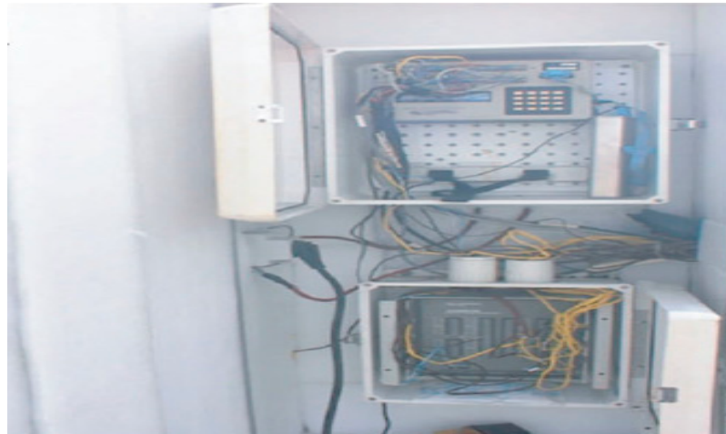
Figure 3. CR5000 data acquisition unit.
