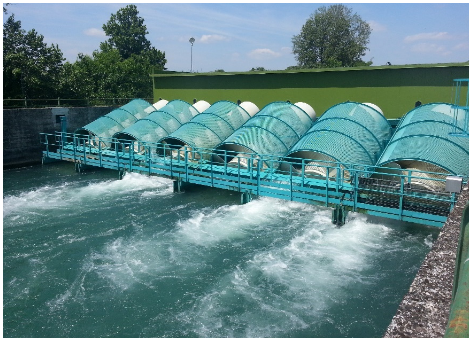
Figure 15. Marengo multi-AST hydropower plant in Goito, Italy [109].
