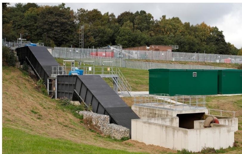
Figure 8. Yorkshire Water's Esholt wastewater treatment AST hydropower plant [73].
