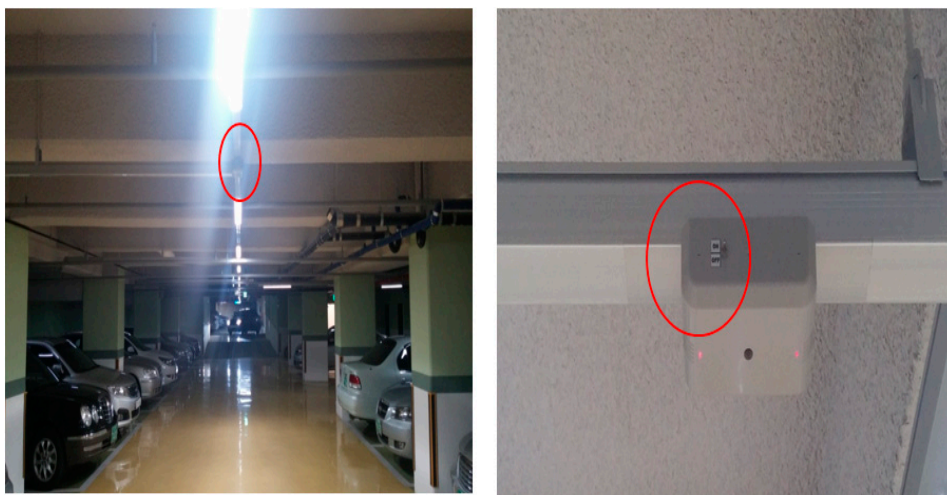
Figure 5. Underground parking space with motion detection sensor installed in ceiling.
