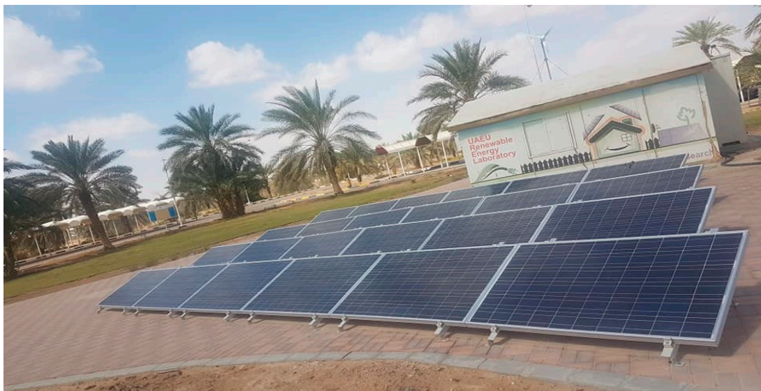
Figure 1. Photovoltaic modules array installed at UAE University, Falaj Hazza Campus.
