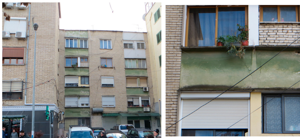
Figure 3. A sample initial occupancy damage state for URM buildings from 2019 Albania earthquake (taken by authors).
