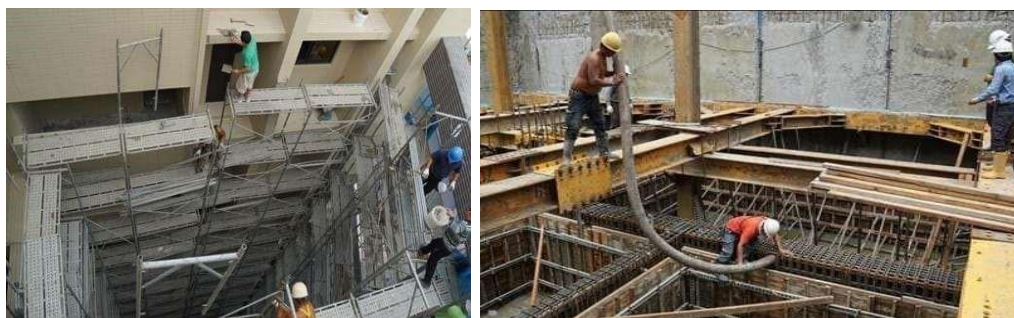
Workers in aloft activities without any protection
