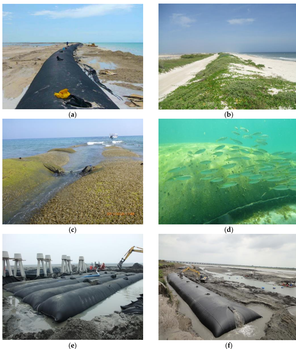
Figure 1. Implementation cases of geotextile tubes (photos copyright by ACE Geosynthetics Enterprise Co., Ltd., Taichung, Taiwan, used with permission). (a) Using geotextile tubes as the core of sand dunes, (b) Vegetation growing back after installing geotextile tubes in the sand dune, (c) Algae growing on the surface of geotextile tubes, (d) Geotextile tubes as an eco-friendly engineering material, (e) Installing geotextile tubes at a construction site, (f) Using nearby sand or sand slurry as the fill material for geotextile tubes.
