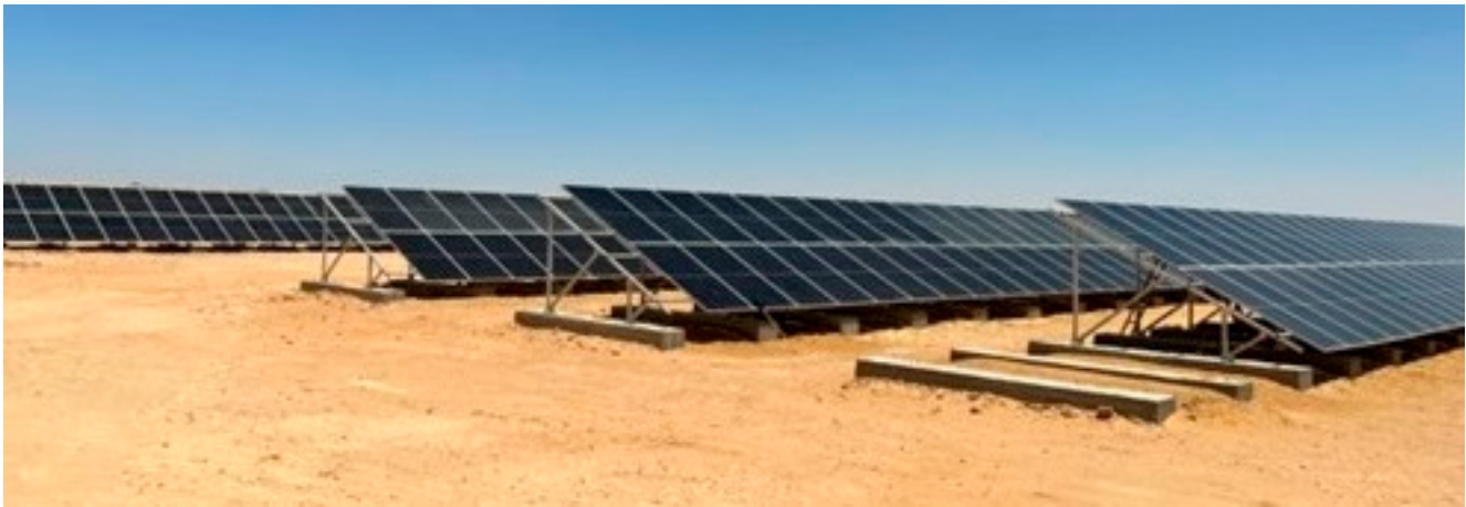
Figure 12. The constructed solar-powered RO desalination pilot plant in El Alamein area.
