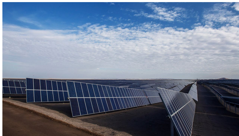
Figure 13. Landscape showing photovoltaic panels in the Panamericana solar facility.
