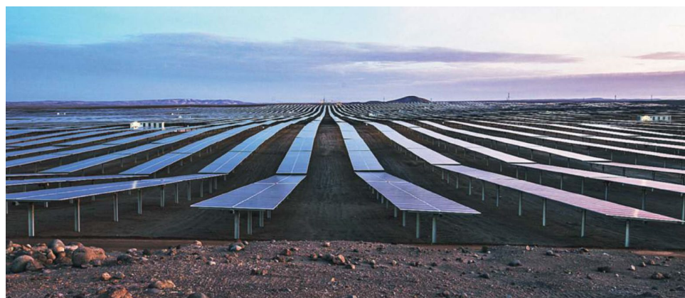
Figure 14. Landscape showing photovoltaic panels in the Moquegua FV solar facility.
