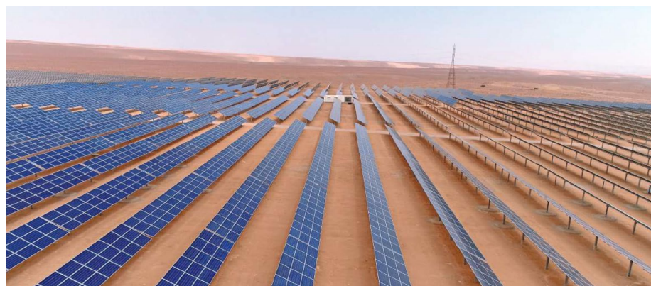
Figure 15. Landscape showing photovoltaic panels in the Intipampa solar facility.
