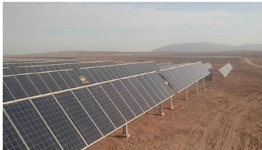
Figure 11. Landscape showing photovoltaic panels in the Majes solar facility.
