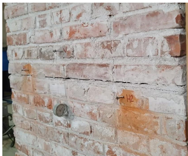
Figure 10. Crack in correspondence to the middle joint.
