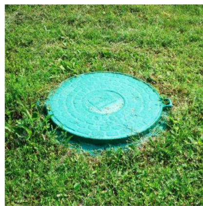
Figure 8. Conventional manhole cover.
