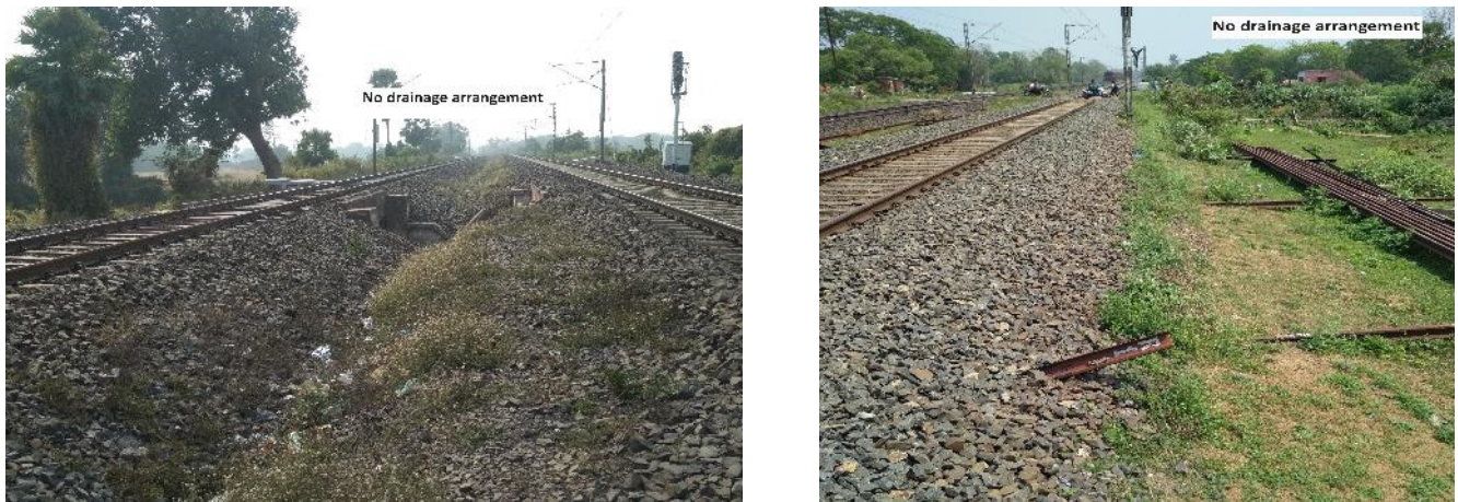
Figure 1. Double-line embankments with no drainage arrangements.
