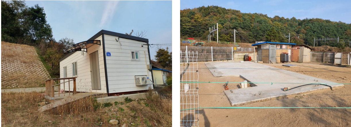
Figure 7. Issue of the high entrance-door threshold (left) and after-treatment of basic placing (right).
