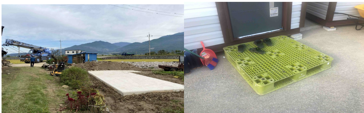
Figure 6. Issues surrounding the height of the entrance door threshold.
