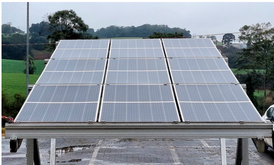
Figure 4. Nine bifacial modules installed in a carport structure. All the modules show some kind of damage to the front and/or rear glass. Image was taken on a day with high humidity, which served as a test for the electrical insulation. It is located in a car park of the laboratories at the Federal University of the Southern Frontier Campus Erechim/Brazil.
