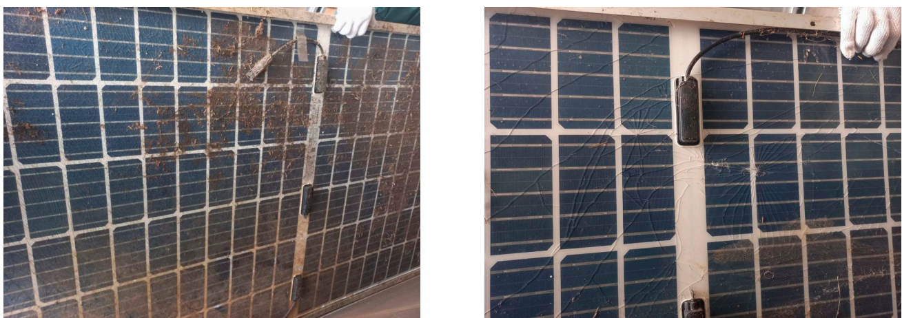
Figure 2. Status of the photovoltaic modules stored after being disposed of at the photovoltaic plant installation site.
