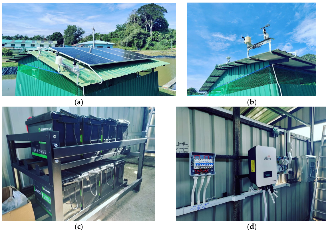
Figure 6. Hybrid PV system: (a) PV array, (b) weather monitoring station, (c) battery storage, (d) hybrid inverter.
