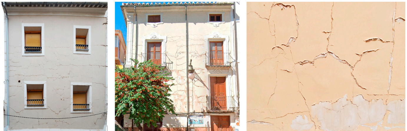
Figure 7. Cracking and peeling of the acrylic paint applied to the gypsum.
