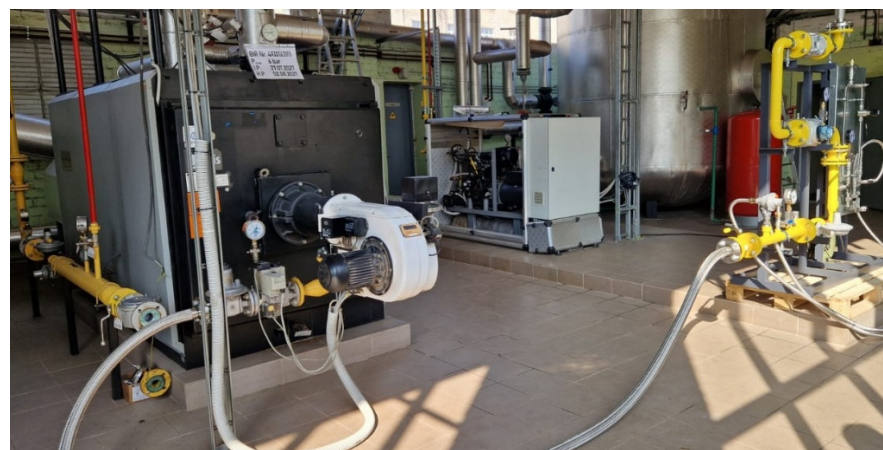
Figure 1. The gas boiler with a hydrogen supply line attachment.
