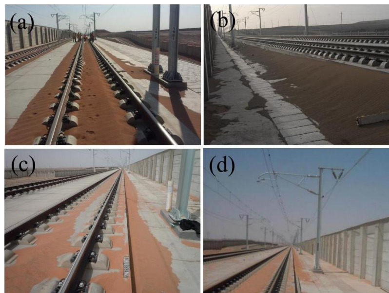
Figure 1. Sand deposition on the leeward side of windbreak walls along the Lanzhou–Xinjiang High-Speed Railway. (a) track sand deposition; (b) railway line sand deposition; (c) track sand deposition; (d) track sand deposition.
