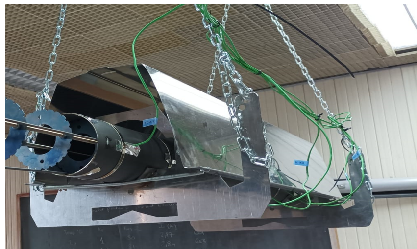
Figure 2. Thermocouple installation along the radiant tube.
