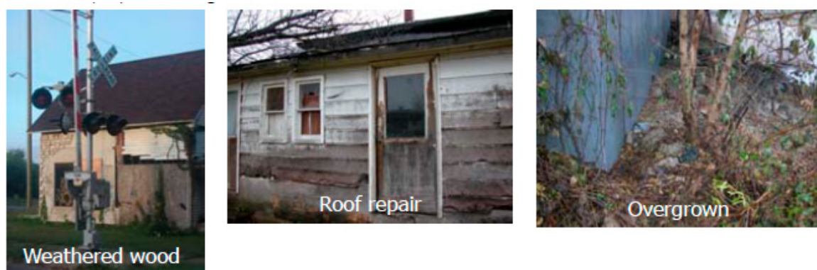
Figure 7. Weathered wood, roof disrepair, and overgrown vegetation provide evidence of neglect in abandoned houses. Photography: K. Sandin.
