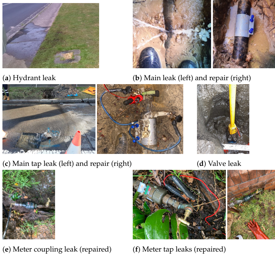
Figure 3. Examples of validated leaks from L&S logger deployments.
