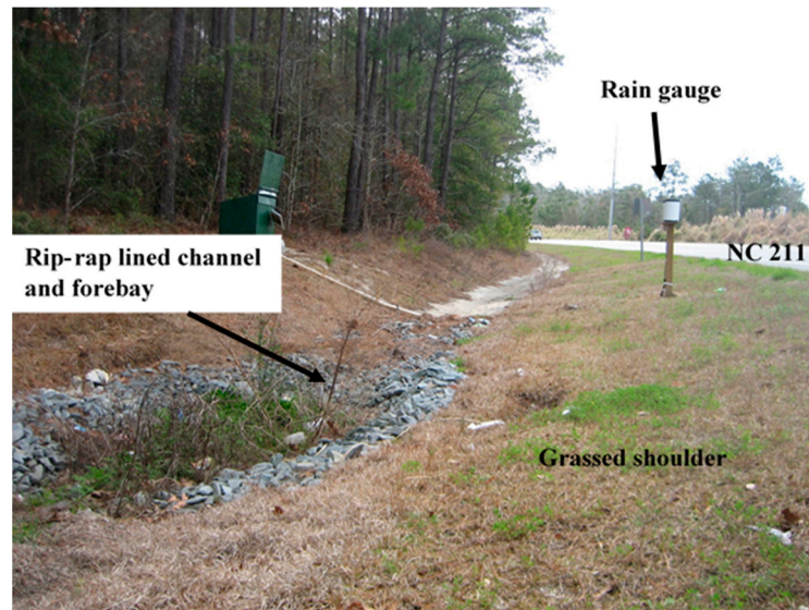
Figure 1. Watershed, grassed shoulder, and rip-rap channel and forebay [47].
