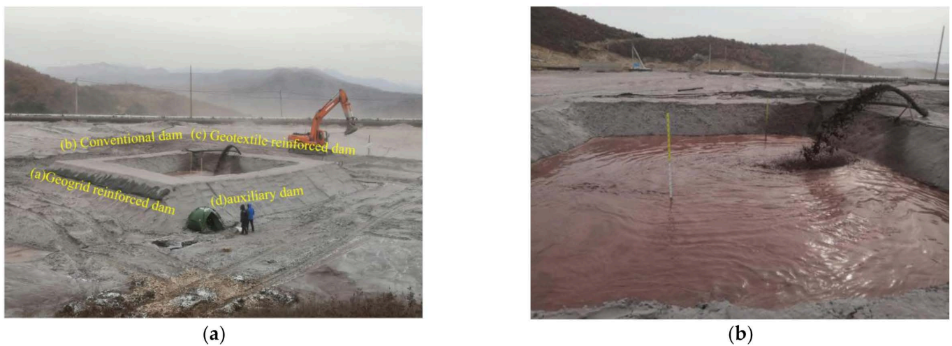
Figure 6. Completion of the overall piling of the reinforced tailings dam and data collection: (a) test dam; (b) water level observation.
