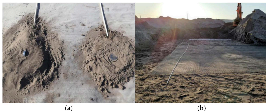
Figure 5. Sensor placement in the dam: (a) pressure box; (b) PWP gauge.
