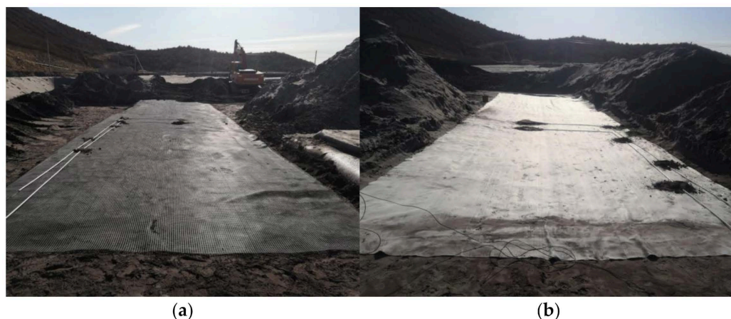
Figure 4. Laying of reinforcement materials for the reinforced dam: (a) geogrid; (b) geotextile.
