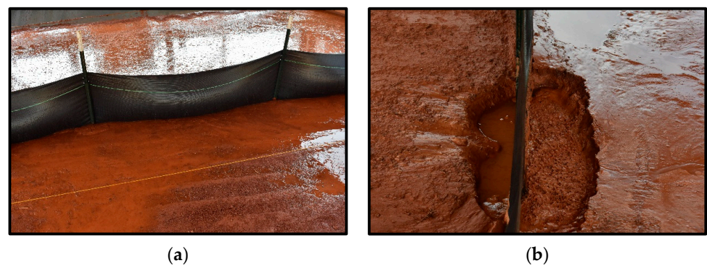
Figure 5. Structural performance of Nebraska DOT standard silt fence: (a) sagging and undermining of silt fence; (b) trench failure of silt fence.
