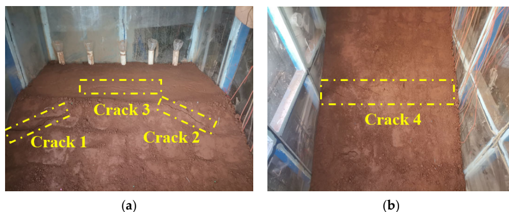
Figure 26. The occurrence of micro cracks on the slope in condition T2. (a) At the top of the slope. (b) In the middle of the slope.
