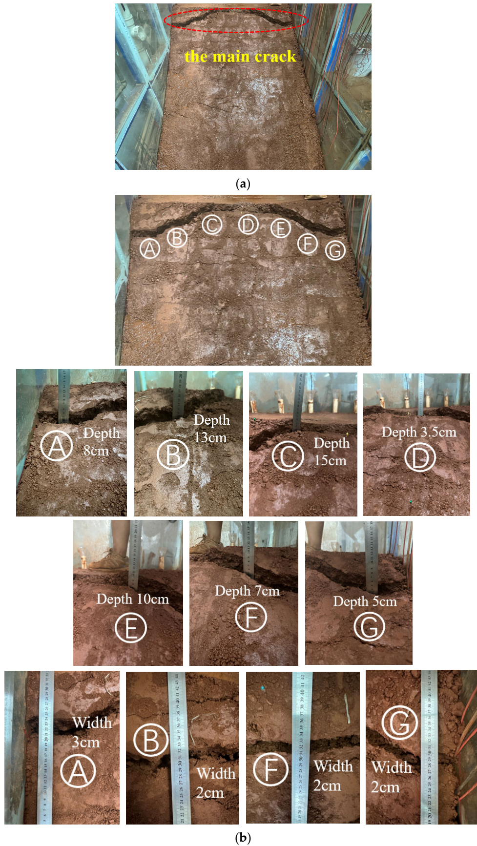
Figure 29. Final morphology of longitudinal cracks in condition T2. (a) Final morphology of longitudinal cracks in condition T2. (b) The depth and width of the final stage of longitudinal cracks in condition T2.
