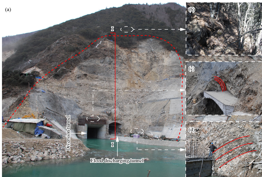
Figure 14. The characteristics of the Laohuzui slope. (a) Overview of the Laohuzui landslide; (b) crack at the rear edge of the slope; (c) flexural toppling phenomenon at the top of diversion tunnel entrance; and (d) flexural toppling phenomenon outside the inlet of the flood discharging tunnel.
