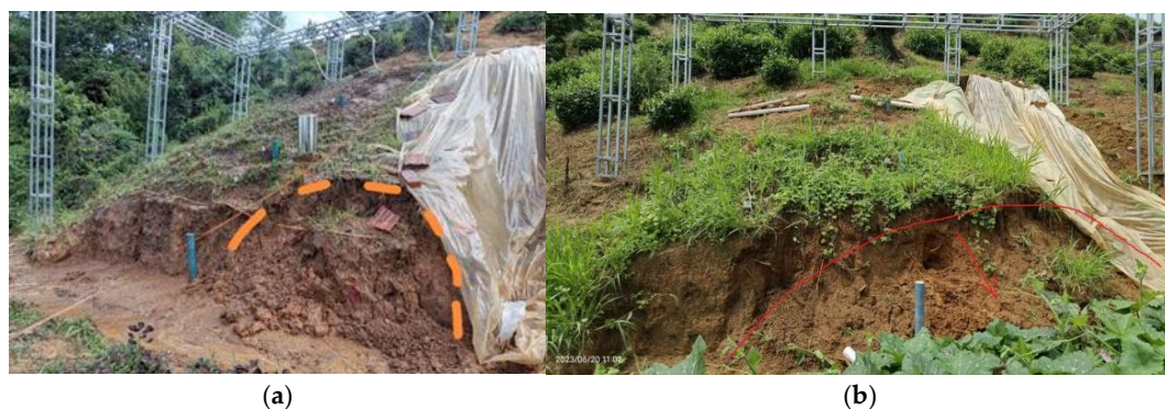
Figure 11. Local slide failure of slope foot during the rainfall process ((a) 10 h of continuous heavy rainfall; (b) after heavy natural rainfall).
